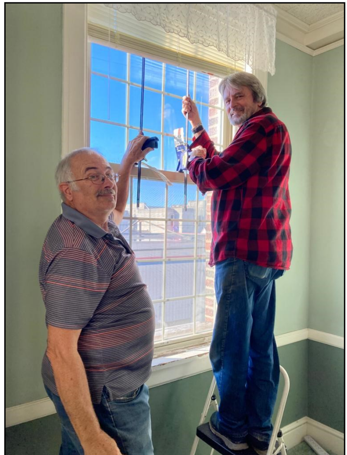
Rex Lane and Terry Ivey show their love by ensuring all the windows in the church are sealed and ready for the winter cold. Sainly Stewardship!!
